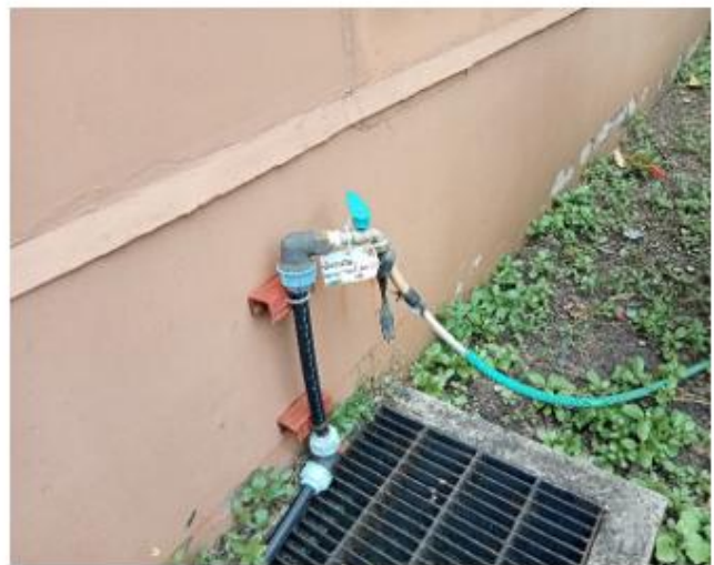
Faucet of water from water recycling
