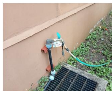
Faucet of water from water recycling
