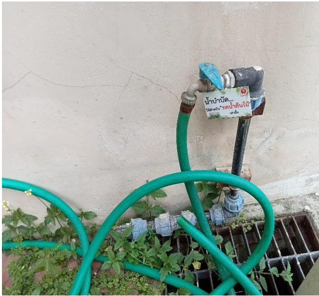
Treated wastewater (effluent) faucet from wastewater treatment system
