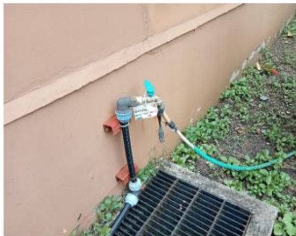
Faucet of water from water recycling
