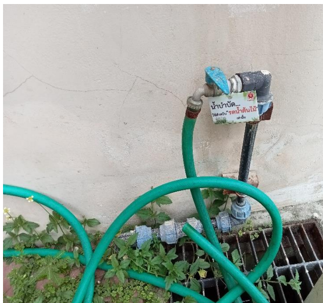
Treated wastewater (effluent) faucet from wastewater treatment system
