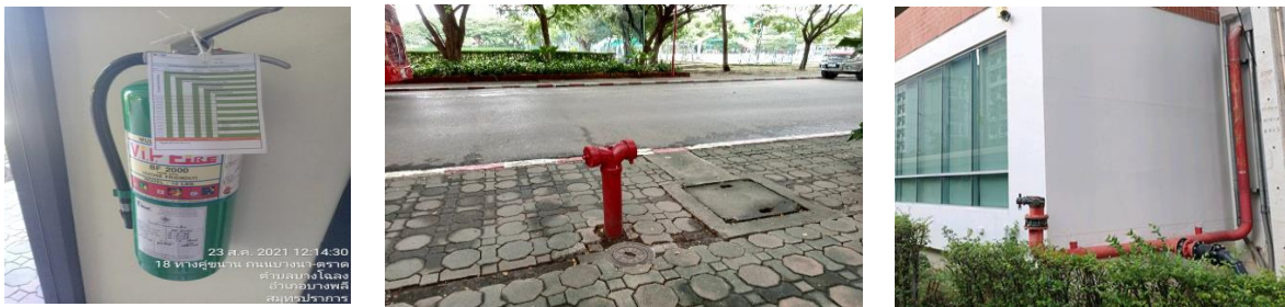
Figure 14 Fire extinguisher, fire hydrant, and fire department connection
