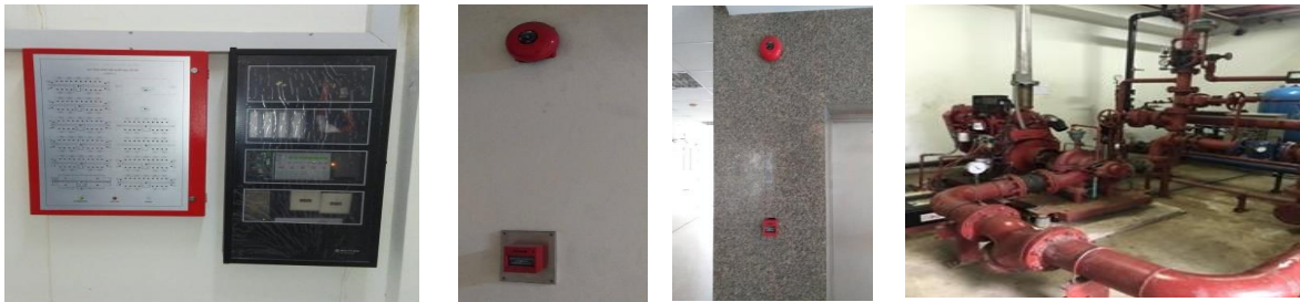
Figure 13 Emergency alarm button and engine fire pump
