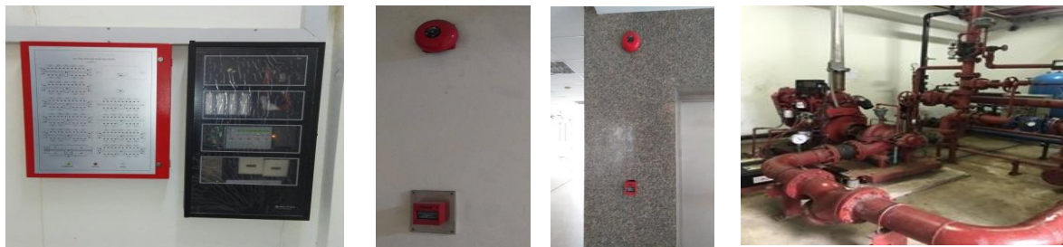
Figure 12 Emergency alarm button and engine fire pump
