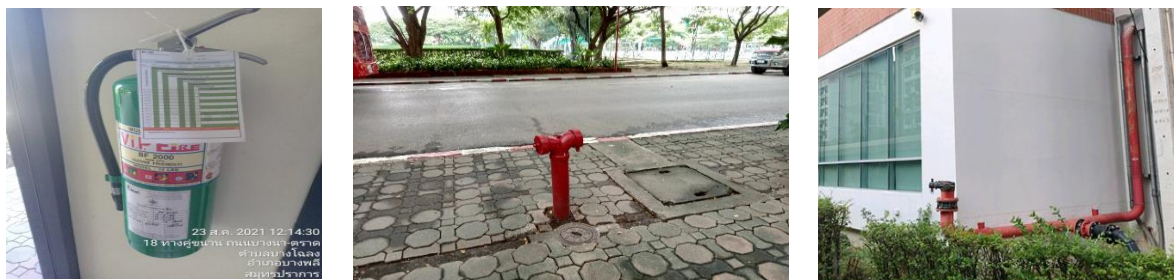
Figure 13 Fire extinguisher, fire hydrant, and fire department connection
