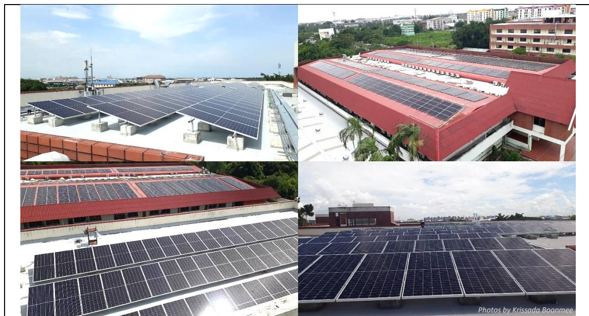
Figure 4 HCU Solar Rooftop Project
