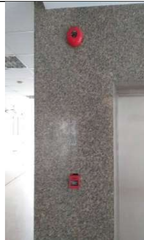
Figure 16 Emergency Alarm Button
